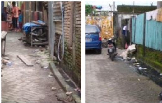
Fig. 5 Gutter and footpath: the narrowest and shallowest sewer in the settlement, this condition can not accommodate the volume of dirty water environment.
